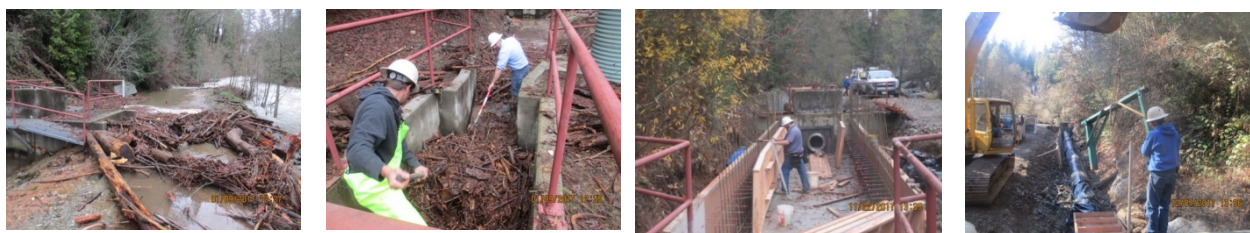
Before (2 left): Newtown Canal is filled with debris in January 2017. And (2 right): NID crews work in late 2017.
