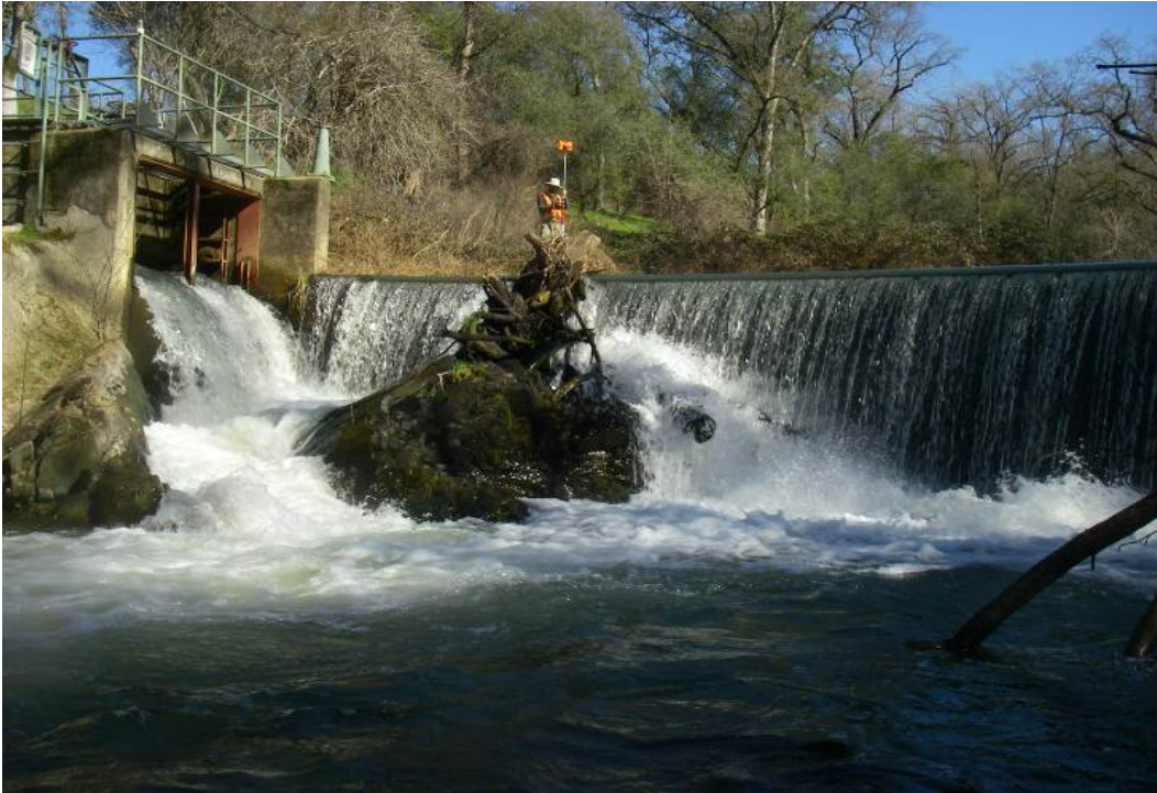
Figure 6.5.3-23 NID Auburn Ravine I Dam and upper end of NID Ditch. Dam height is about 11 feet. (Flow pictured is approximately 110 cfs. No diversion to Auburn Ravine I canal is occurring at this time and water at the head of the canal is being returned to Auburn Ravine at the left of the photograph.)
