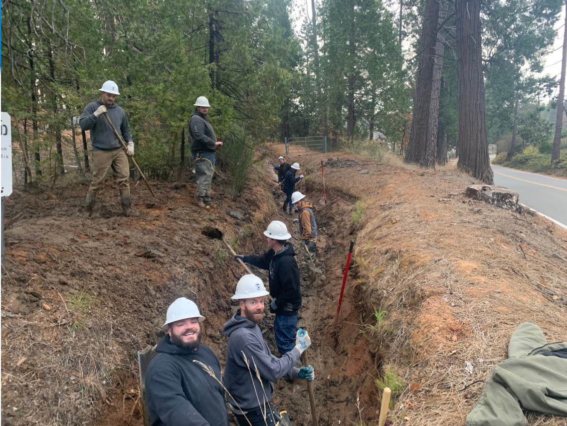
Preparing a canal for the start of irrigation season, which began on April 15: (In the canal L-R) Utility Workers Davin Chittock, Patrick Sheehan, Daniel Roth, Zachary Clark Ware, Wyatt Landrum, Adam Custer and Joe Amberg; (On the berm) Sean Rash and Joe Franks.
