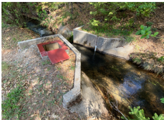
Lower Grass Valley Canal Head Gate/Gaging Station
