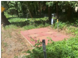
Silver Way PRV Underground vault PRV
