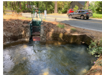
Lower Grass Valley Canal Head Gate
