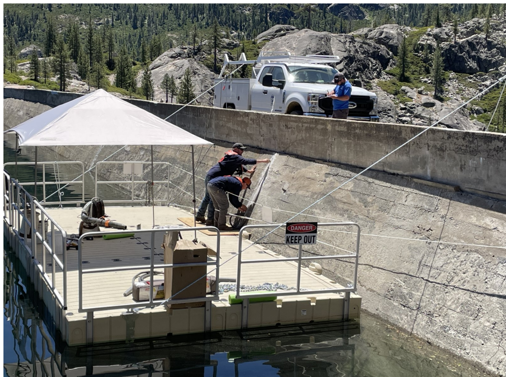
Hydropower workers use a floating dock to make routine surface repairs on the Bowman Dam.
