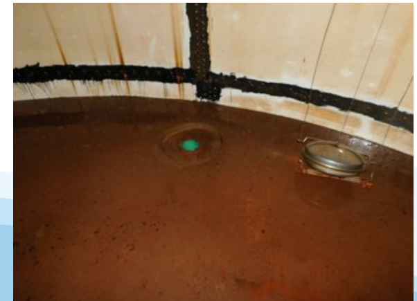
Rusted Wall Inside Tank
