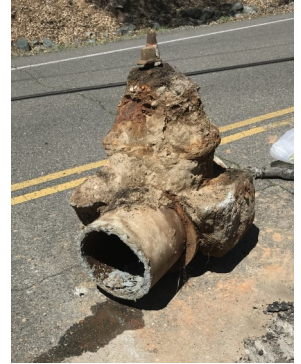
You can see the ring of asbestos on the AC pipe where the crew cut out the old hydrant.
