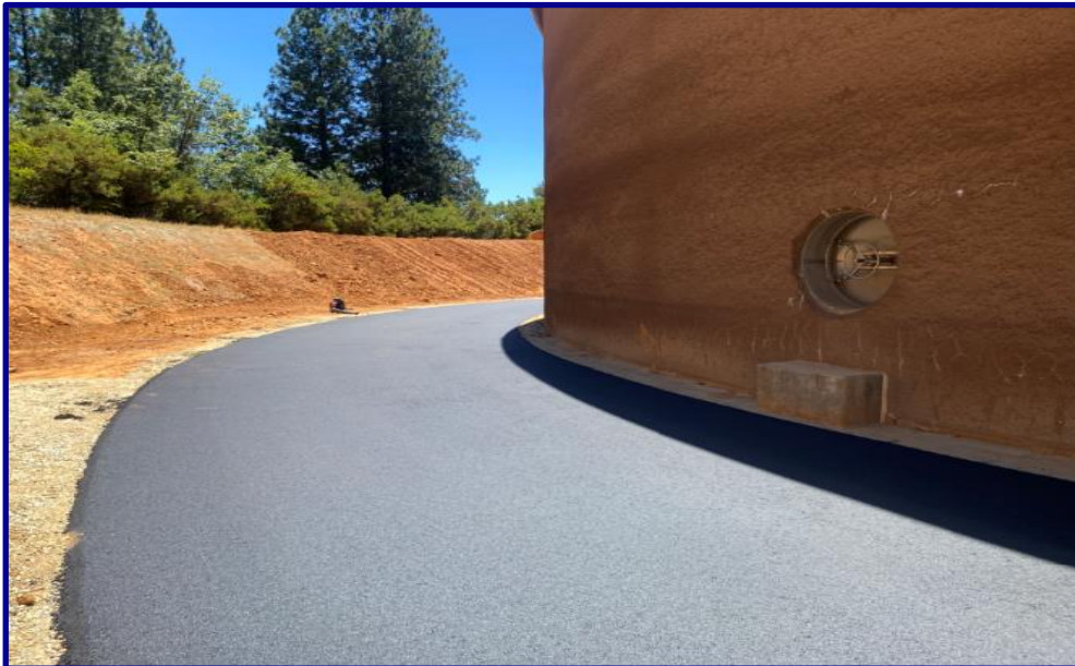
Side view of water tank
