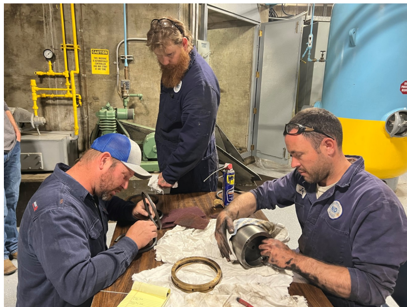
An NID hydropower crew takes advantage of the unexpected outage of the South Yuba Canal to complete maintenance at the Dutch Flat #2 Powerhouse.
