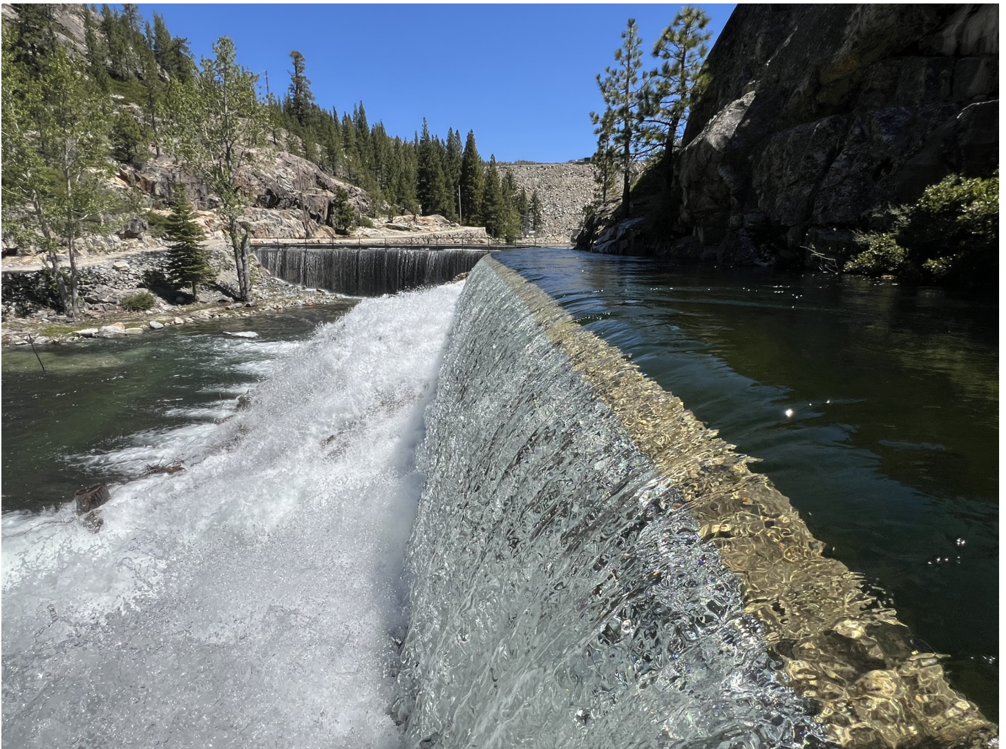
Snowmelt at the Canyon Creek Diversion Dam, Head of the Bowman-Spaulding Canal, and Bowman House.
