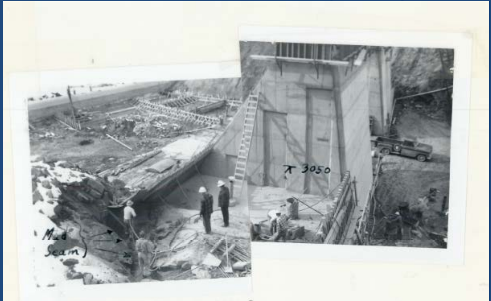
Raised Spillway Crest and Concrete Apron of Upper Plunge Pool built to modern standards, 1964
