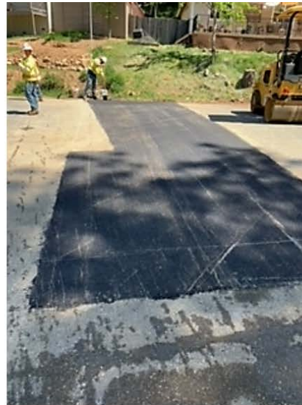
Final “patch paving” – One of the larger roadway patches in Lake Wildwood.
